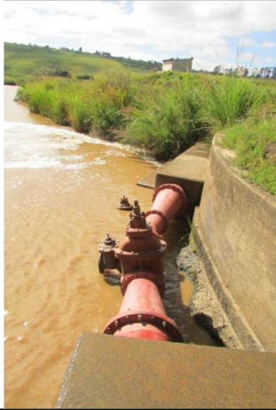
Figure 6.15: Abstraction pipeline infrastructure on the downstream side of the road bridge.
